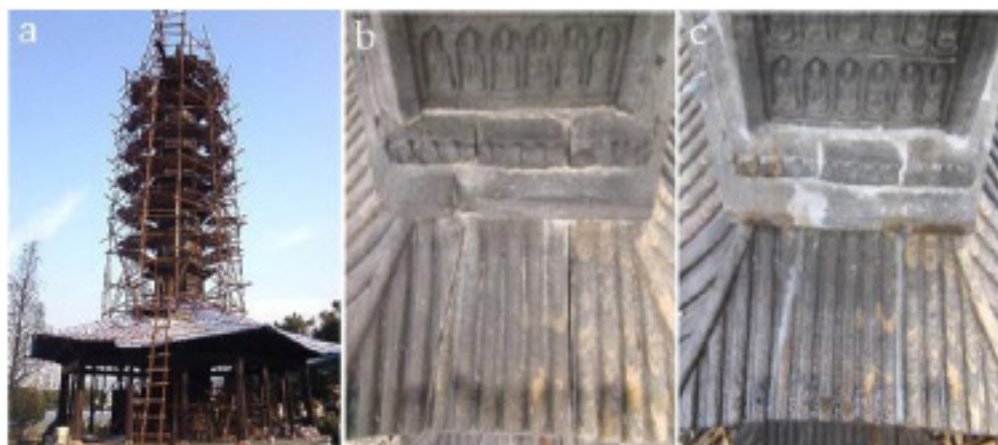
Figure 2: a Guoan Temple Tower restoration site; b and c Fourth eaves of pagoda before and restoration [1]
